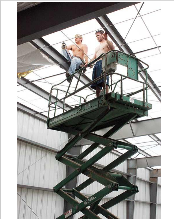
Garrett Palawski, left, and Josh Winter, both of Chanute, ride atop a construction lift inside the building going up for RobotZone east of the Winfield Industrial Park. Both men work for Brown Construction of Chanute. (Dave Seaton/Courier)
